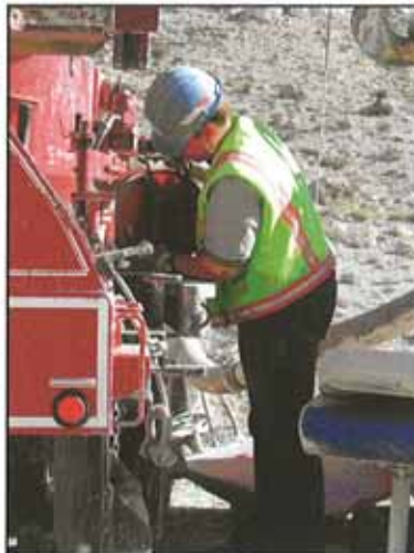
Readings taken by Anna Draa following installation, showed the static water level at 770 ft bgs.
